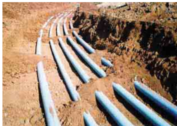
PVC Pipe for water supply
